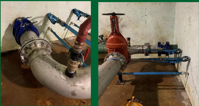
Coupler was replaced and temporary supports added for additional reassurance for over the Christmas break.
